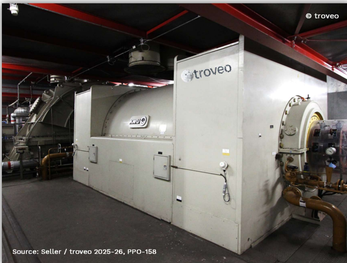
power generator set and steam turbine (in the back)
