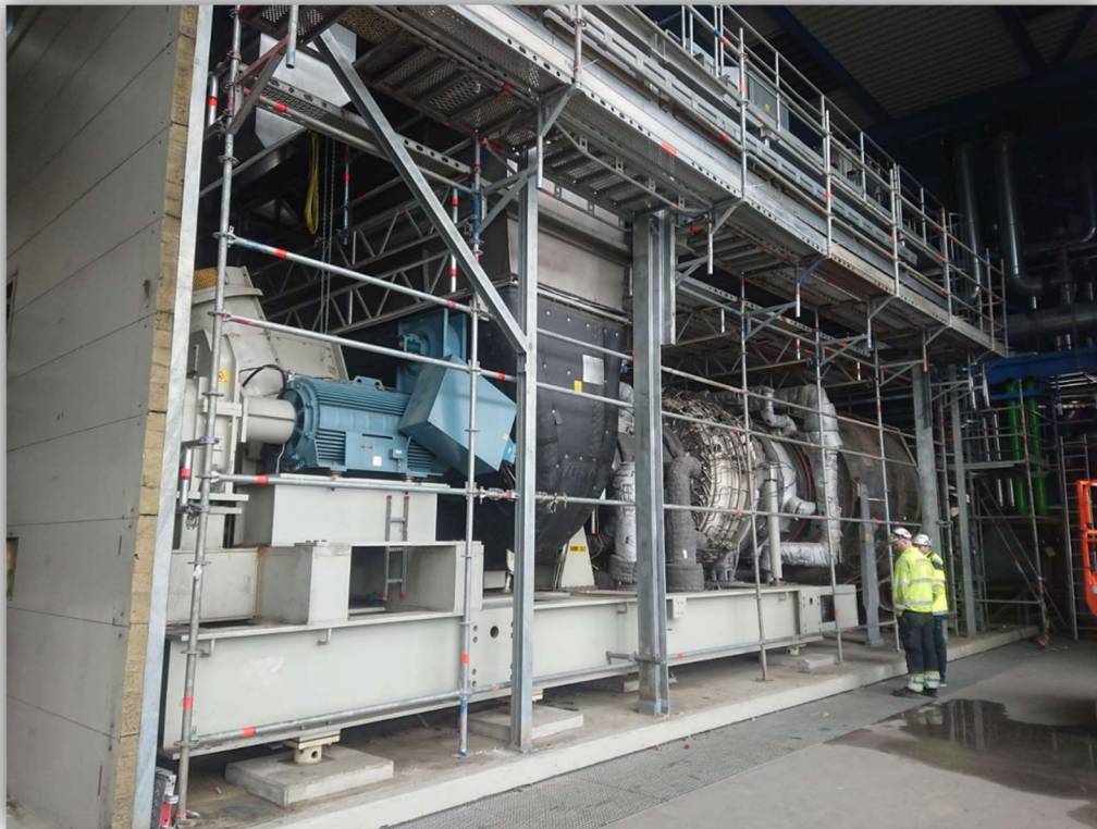
Gas turbine – Turbine and generator after opening of canopy cover
