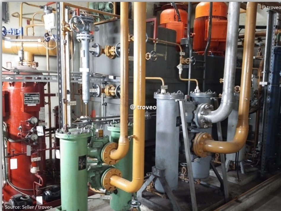
steam turbine – bearing oil lubrication system
