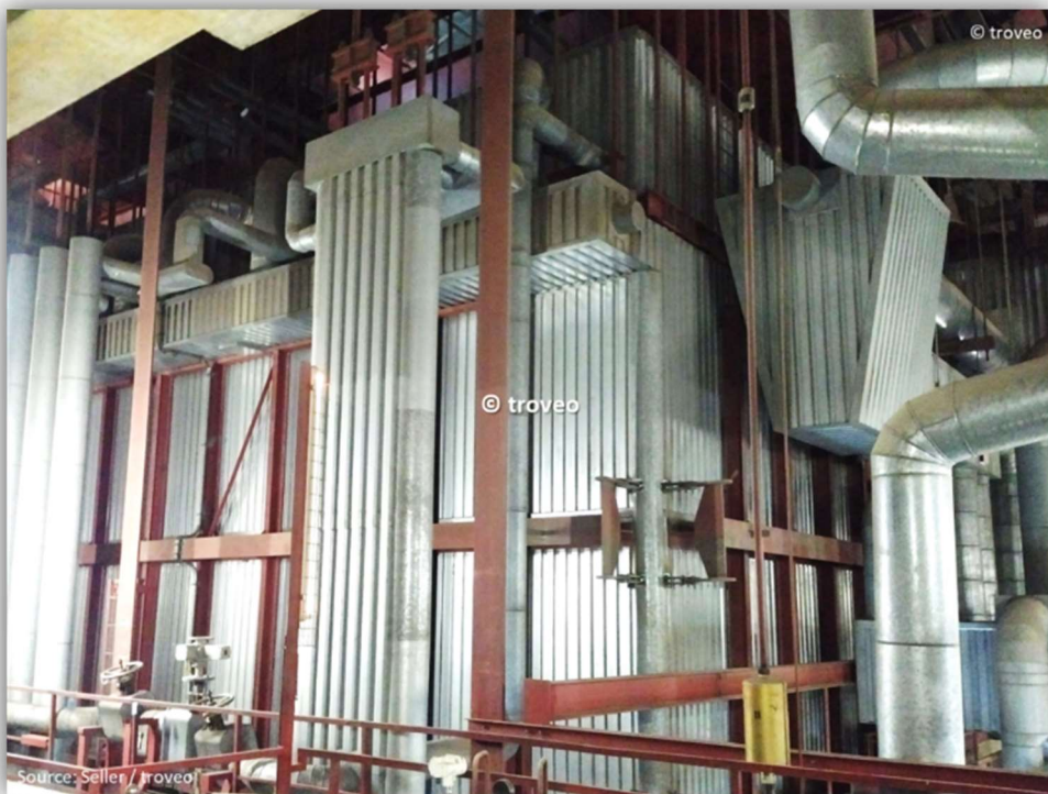
steam boiler – boiler top-side suspension
