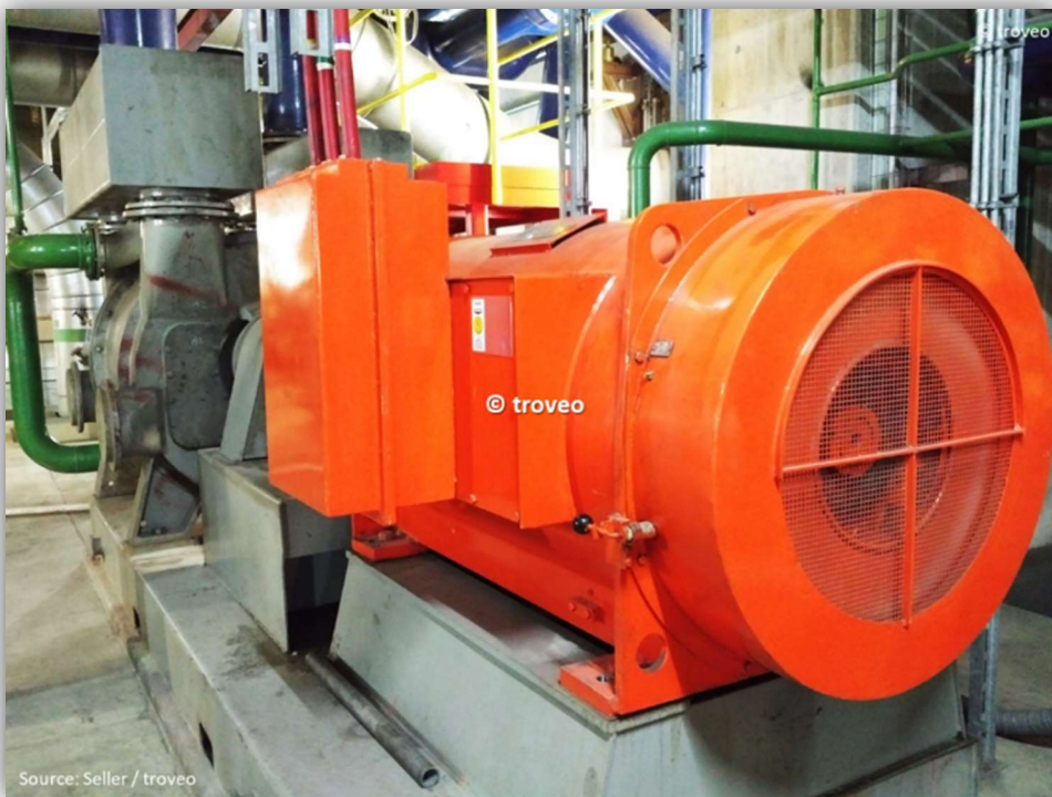
cooling water system – loop pump
