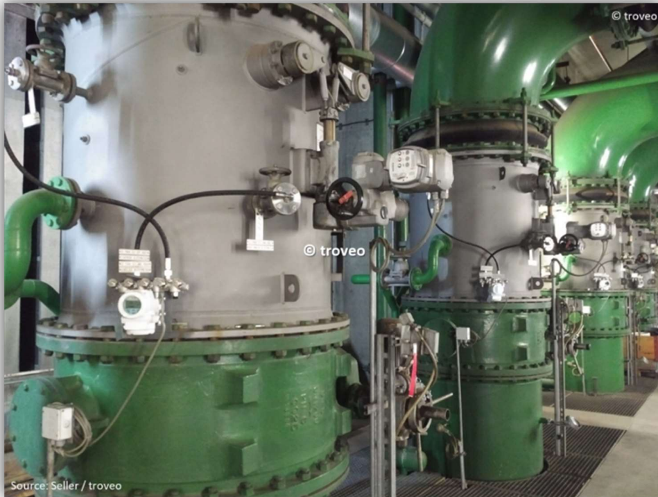
water/steam cycle – high-pressure condensate pipes
