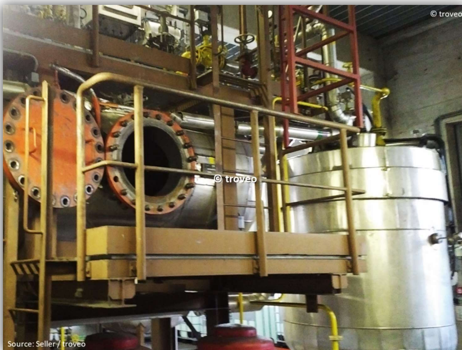
flue gas cleaning system - ammoniac evaporator station for the DeNO x filter
