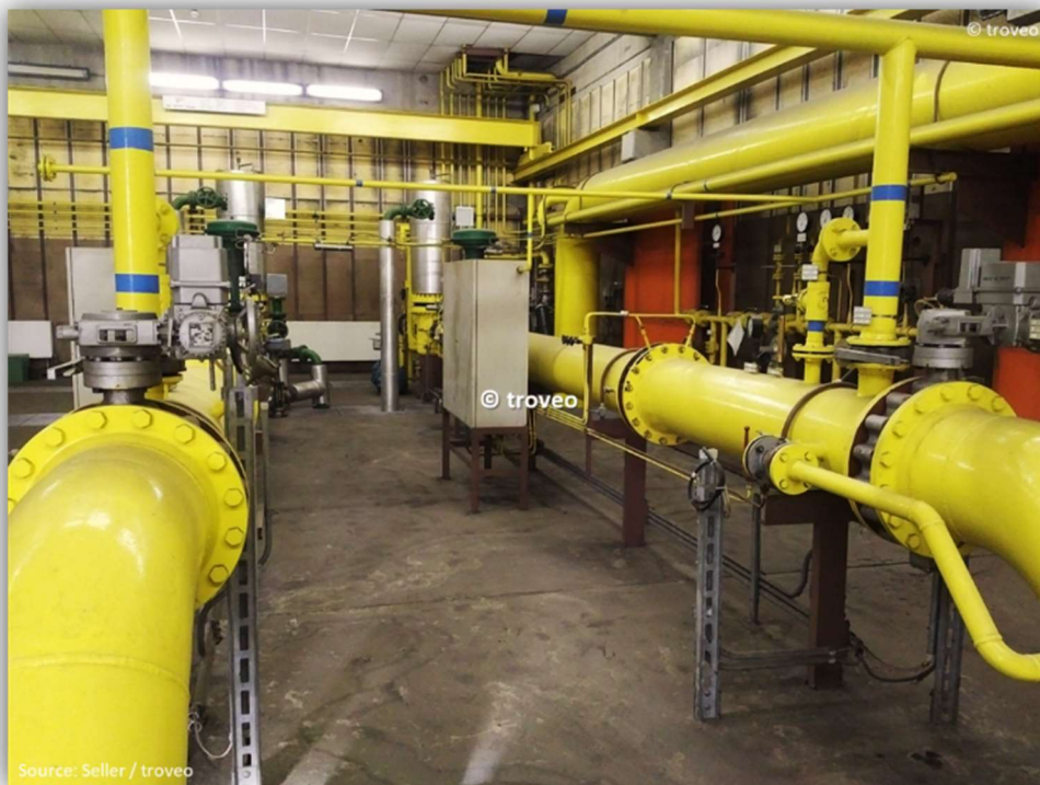
fuel supply - gas pressure reducing station
