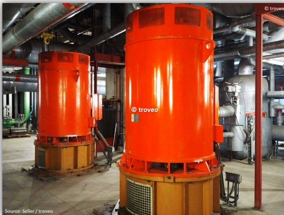
water/steam cycle – main high-pressure condensate pumps
